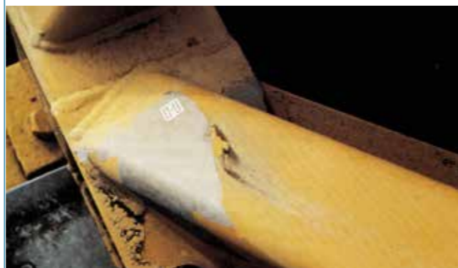
Fig. 11-3. Poor adhesion of a yellow high-gloss alkyd topcoat over a grey chlorinated rubber based primer. The primer adheres excellently to the galvanized steel, whereas the alkyd topcoat does not adhere to the primer (22).
