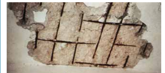
Fig. 10-14. Spalling of cover layer over reinforcement in basement, due to the corrosion of reinforcement bars.
