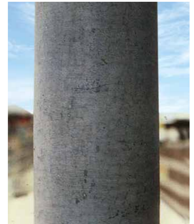
Fig.10-1. Exposed surface of a zinc coating with outer layer of pure zinc. The shiny surface disappears to be replaced by grey corrosion products (sometimes called zinc patina).
