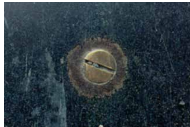
Fig. 10-13. Brass bolt in hot-dip galvanized steel on a parking deck.
