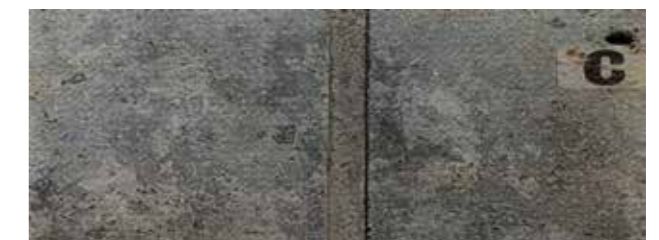
Fig. 10-11. 6 mm-wide milled groove through 60 µm thick zinc layer on steel exposed for 5 years in severe industrial-marine environment in Holland. Note the coating of zinc salts in the groove, and the total absence of rust breakthrough. (J F H van Eijns-bergen).
