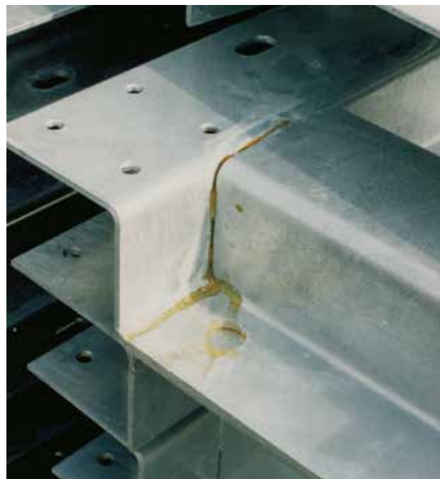
Fig. 7-11. Acid trap where the acid has corroded through the zinc coating, which leads to discolouration of the surface.
