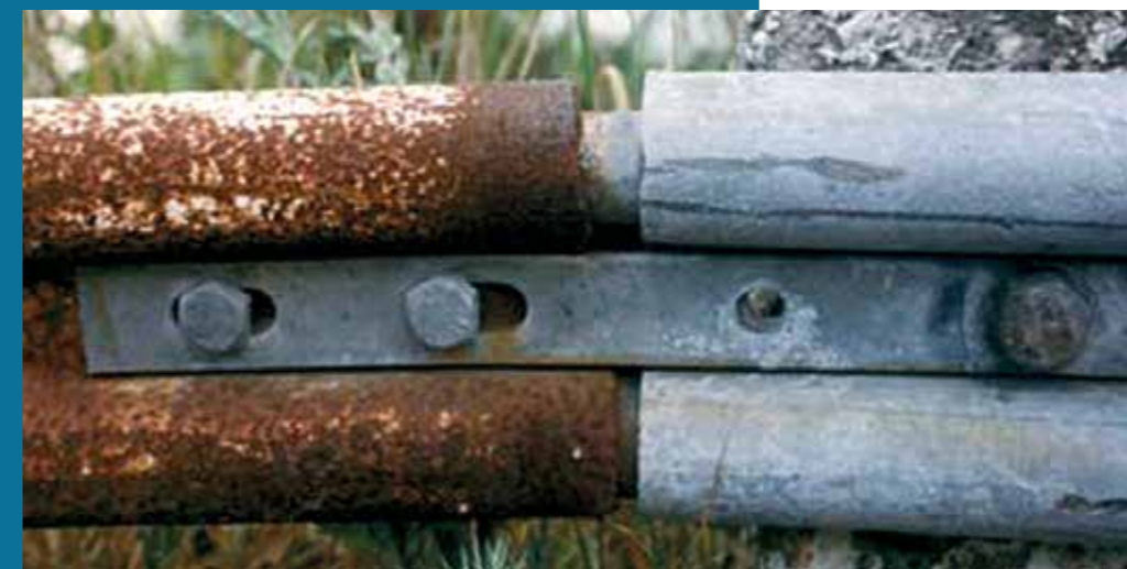
Fig. 1-2. On the left, a painted fence that has corroded. Compare with the hot dip galvanized fence on the right.
