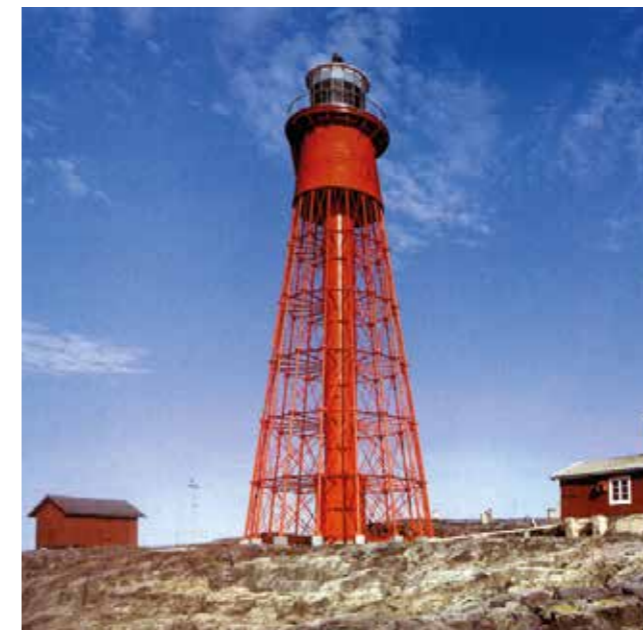
Fig 11-1. The lighthouse Pater Noster is one of the first duplex treated steel constructions in Sweden. It was galvanized 1868, and after that painted
