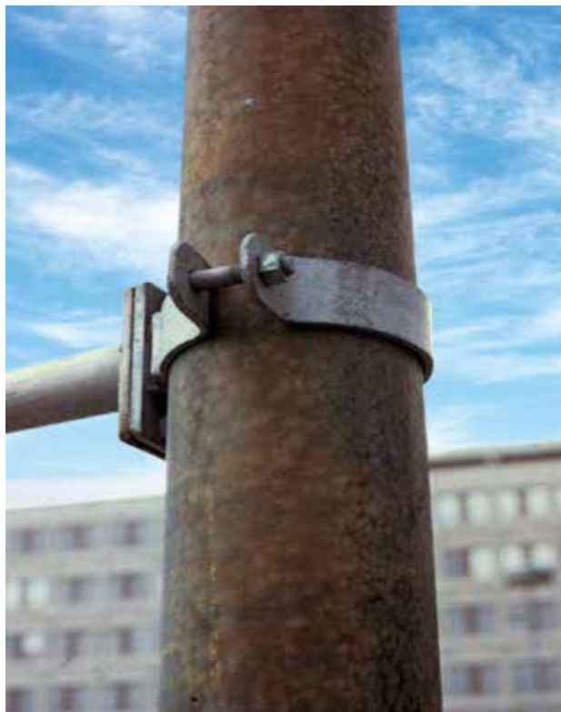
Fig. 10-2. Discoloured surface on lighting column.
